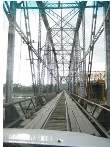
Fig. 2 Poor road infrastructure
