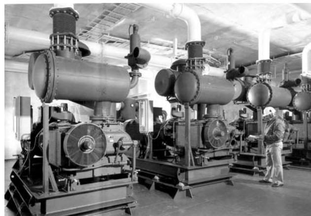
(Fig. 7 Compressor room)
